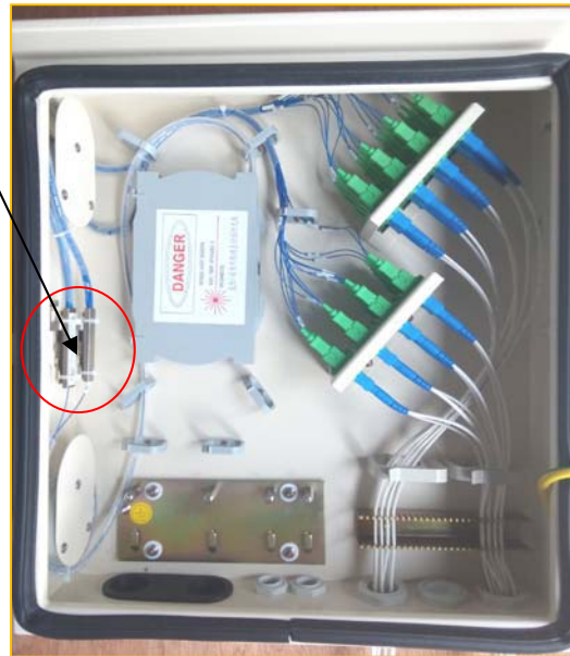
Optical Splitting Box
